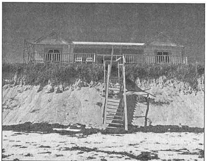
Figure 9. House on nearby Guana Cay in danger of imminent collapse (Photo: Sealey)
